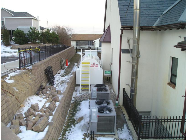
Fuel tank with ladder, between two retaining walls and the church building. Air conditioning units are to the forefront.
